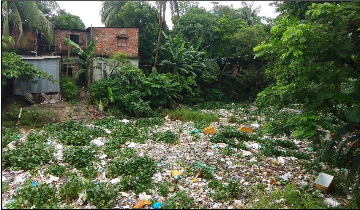
Figure 5: Shuvaddya Canal which needs to restoration
